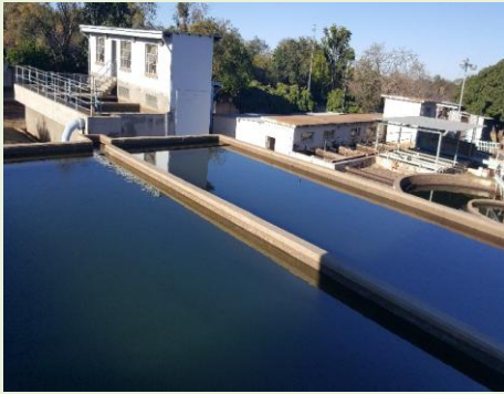
Bela- Bela Water Works
