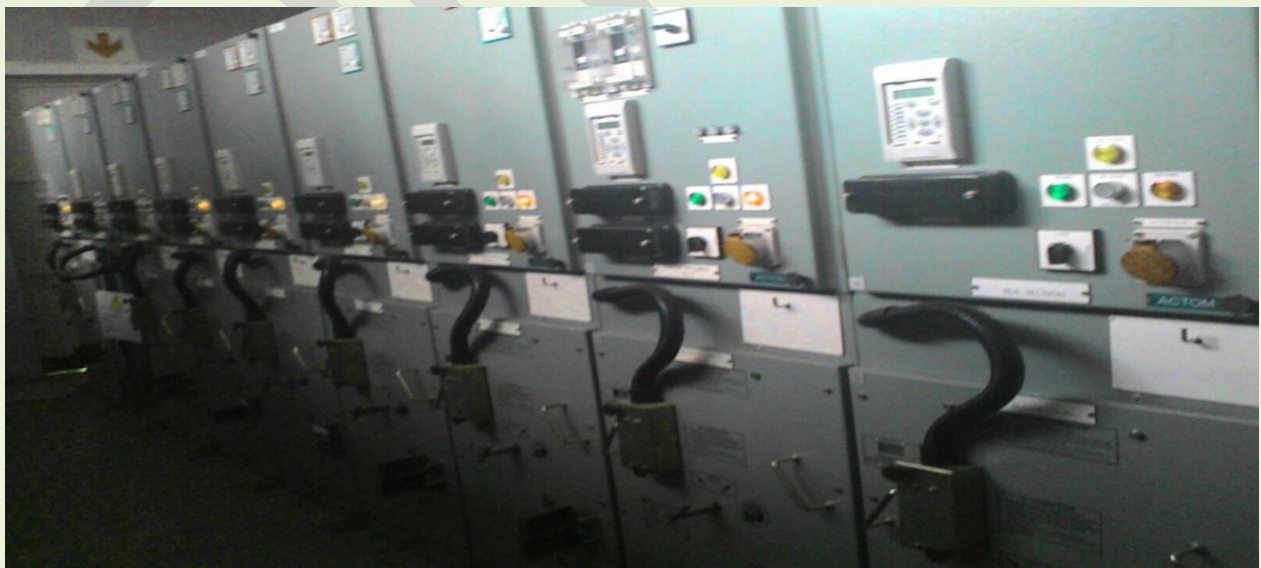
FIGURE: 4 BELA-BELA SUB STATION
